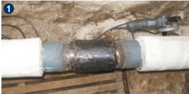
1 Pipe preparation as per GW 15, clean, dry and free of grease. If shrink sleeves are used, preheat to 70°C.
